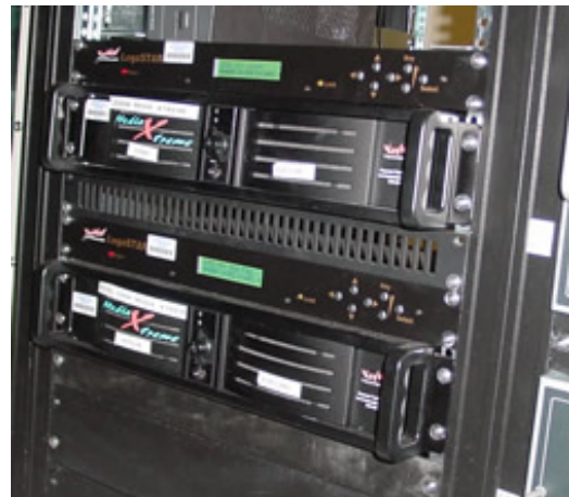
The MediaXtreme in the racks at Cox Cable.
